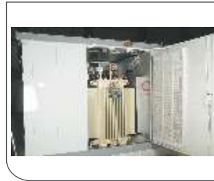
CSS - TRANSFORMERS SIDE
