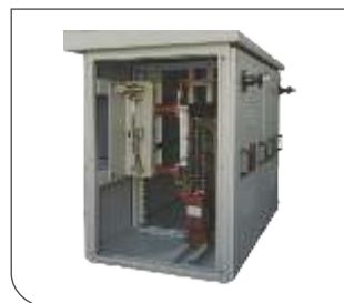
NEUTRAL GROUNDING RESISTORS
