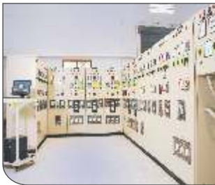
MOTOR CONTROL CENTERS
