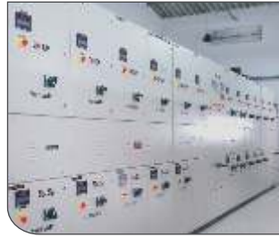
MOTOR CONTROL CENTERS
